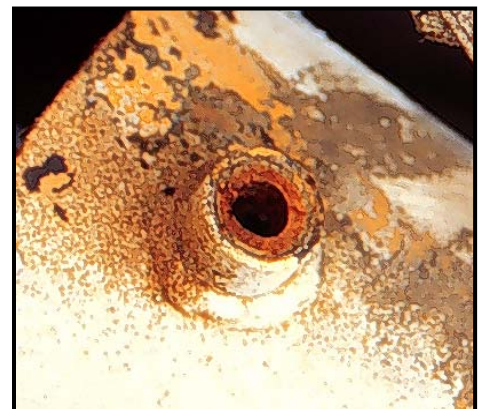
Photo 3 -- Hydraulic line input showing broken edge of nipple. Photo taken several months later shows significant additional rusting.
